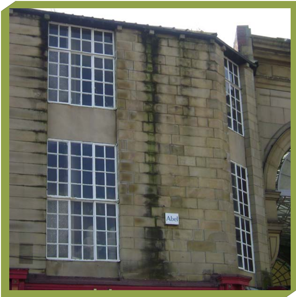
OVER TIME, A DRAINAGE PROBLEM WILL RESULT IN THE GROWTH OF ALGAE ON WALLS.
