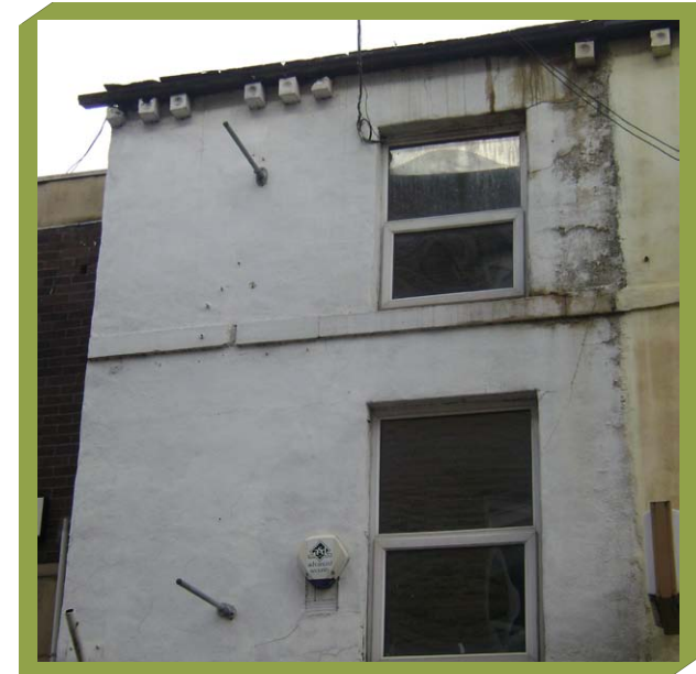
SIGNIFICANT DAMAGE CAN BE CAUSED TO WALLS IF WATER PROBLEMS ARE NOT RESOLVED EARLY.
