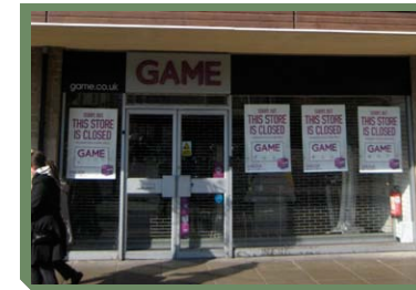
INTERNAL OPEN MESH SHUTTERS LOOK BETTER EVEN ON SHOPS THAT HAVE CLOSED.
